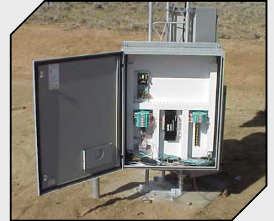
M2M iGateway's link wells by solar powered radios NEMA-4 enclosures endure extreme exposure to the elements
