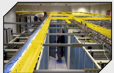
M2M data center hosts the application and data, and around-the-clock monitoring from a network operations center ensures maximum availability, backup, and automatic recovery – providing the basis for guaranteed service.
